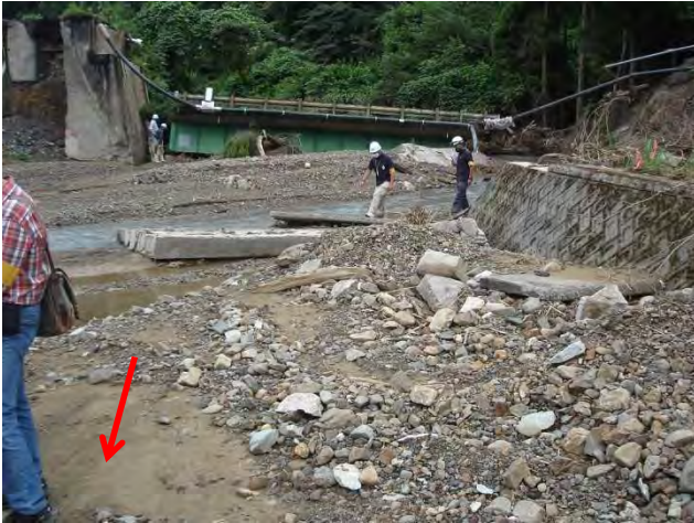
写真-9 左岸側護岸の流失
