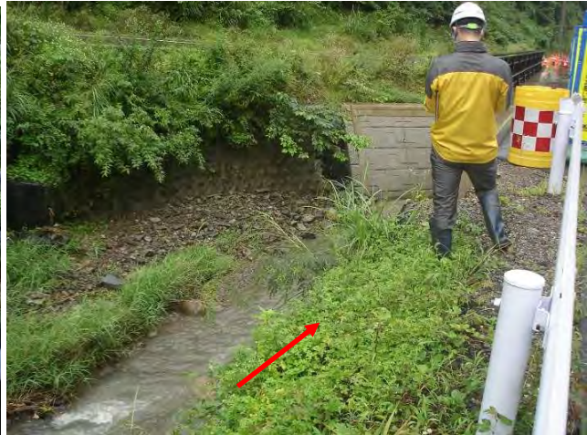
写真-7 左岸洗堀
