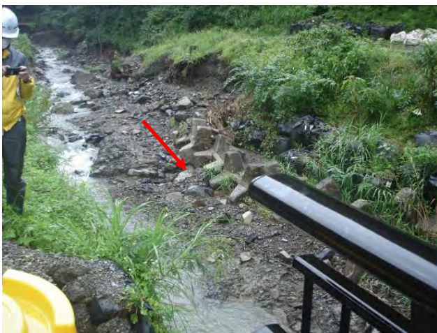
写真-6 左岸洗堀
